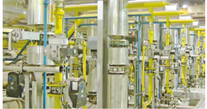
Walking beam furnace with overhead firing
