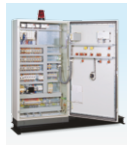
TC 4 installed separately from the system in a control cabinet
